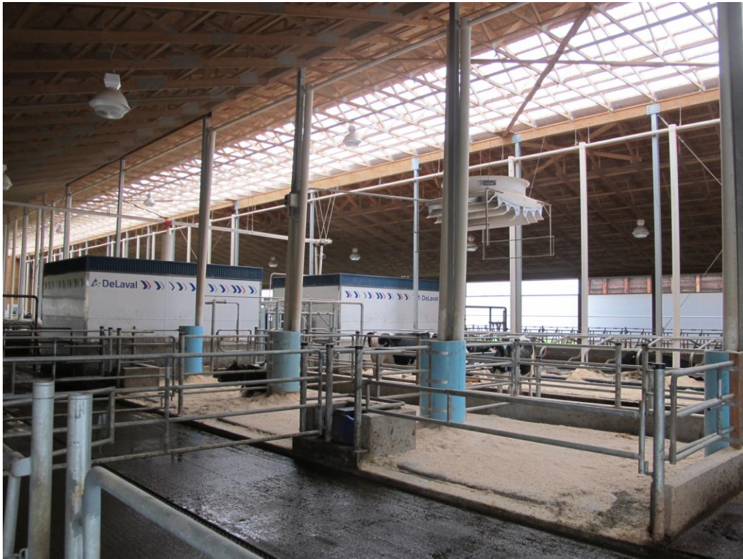
Flex augur shavings delivery to pens (foreground) and stalls (further back on right) at Walrose Farms
