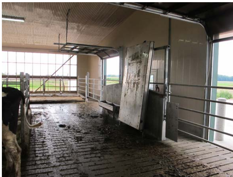
A hinged footbath in a remote crossover can be stored vertically when not in use.
